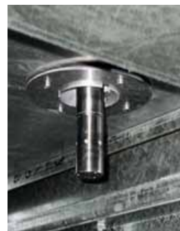
Typical sensor installation
