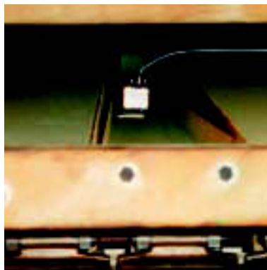
Typical assembly: An HP-250A sensor installed between 2 hot-air ducts
