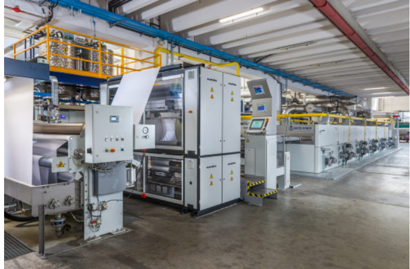
Mahlo combination system with Orthomax RFMB and Optipac VMC process control on a stenter in the finishing area.
