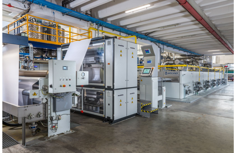
Mahlo combination system with Orthomax RFMB and Optipac VMC process control on a stenter in the finishing area.
